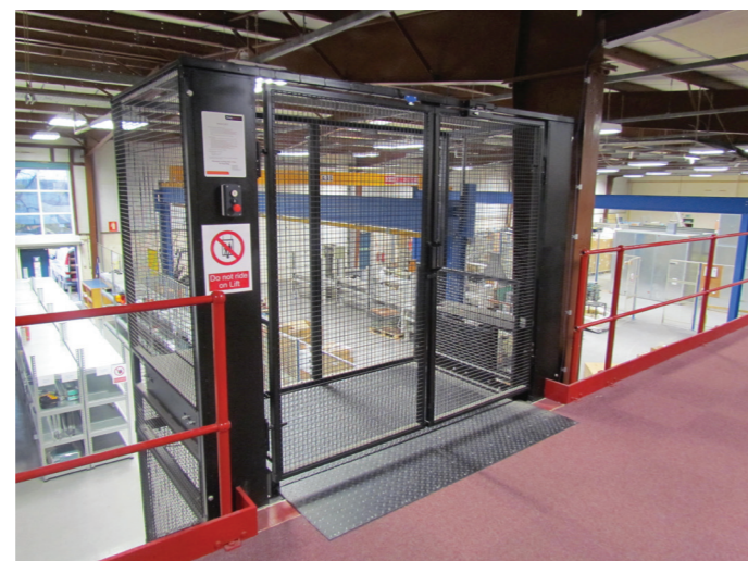
Interlocked gate at upper level
