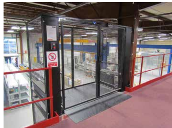
Interlocked gate at upper level
